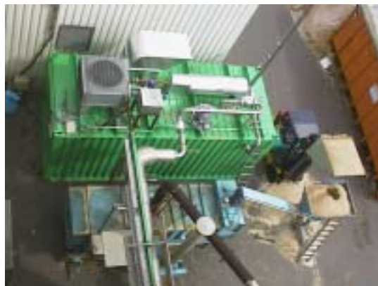
Figure 7: The BHPP-container and the belt dryer for biomass feedstock at the pilot plant in Oberhausen (top view)
