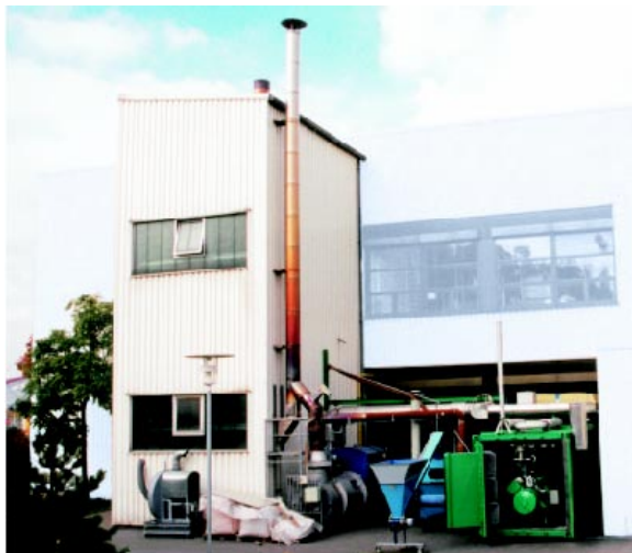
Figure 2: 0.5 MW-Pilot plant at Fraunhofer UMSICHT.
